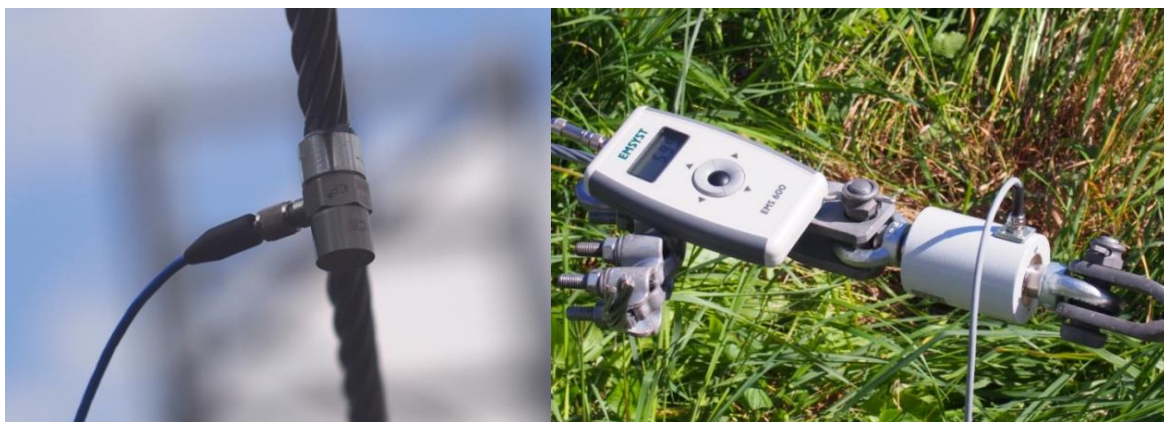
Fig. 2. Piezoelectric accelerometer attached on the power line (left), attaching of the tensometer to sensing the axial force in power line (right)
